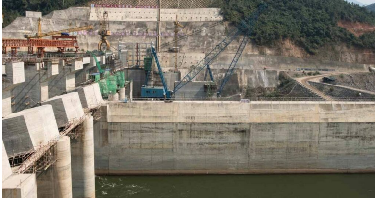
The Nam Ou 3 Hydroelectric dam built on the Nam Ou River in Luang Prabang is part of China's Belt and Road Initiative.
